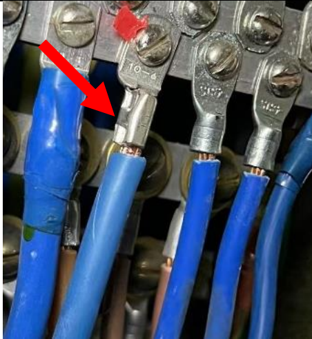
Example 27 : ✗ Lugs are not wrapped with insulating tape
