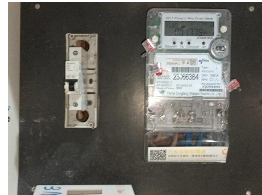
✓ Phase wire should be connected to the Miniature Circuit Breaker (MCB)
