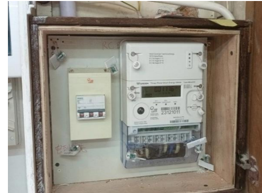
✓ Service-entrance lines of meter should be connected behind the meter board
