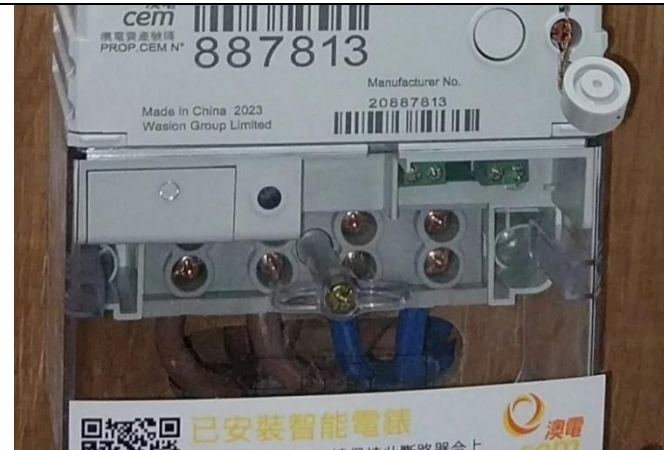
✓ Correct color of single-phase service-entrance lines is brown and blue
