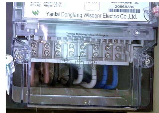
✓ Correct color of three-phase service-entrance lines is brown, black, grey and blue
