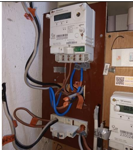
Example 18 : ✗ Meter position and meter board are not securely fixed
