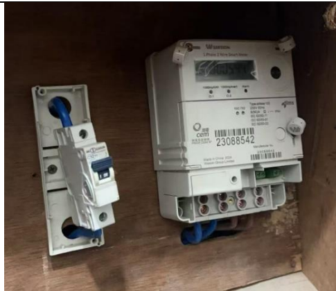
Example 14 : ✗ Neutral wire incorrectly connected to the Miniature Circuit Breaker (MCB)
