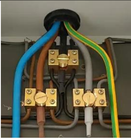
Example 31 : ✗ Incorrect way to connect service-entrance lines
