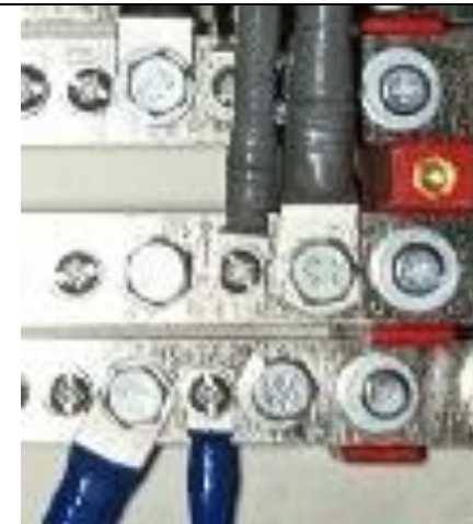
✓ The lugs of service-entrance lines from different units should be connected correctly
