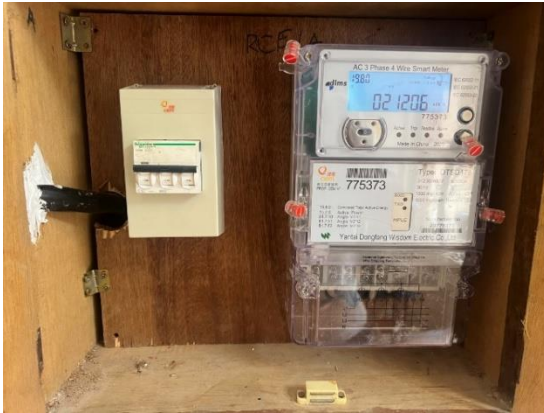
Example 13 : ✗ Service-entrance lines of meter installed in open wire way
