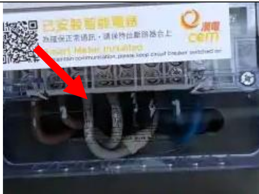
Example 12 : ✗ Incorrect color of three-phase service-entrance lines
