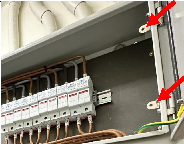
Example 32 : ✗ Incorrect way to install transparent polycarbonate (PC) board
