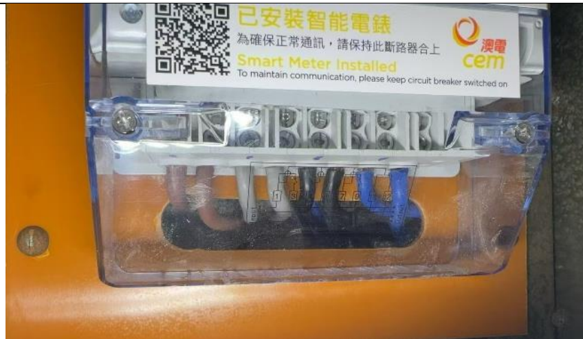
Example 17 : ✗ Incorrect meter wiring sequencing
