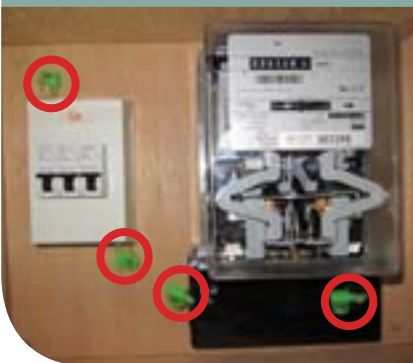
Three-Phase Electromechanical Meter
